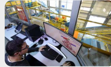
1 AUTOMATIC CONTROL (SCADA) ROOM
